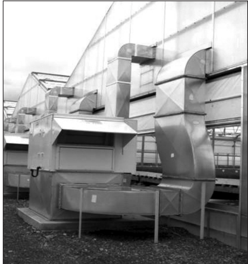
The unit heaters and ducting are located in the back of the greenhouse.
